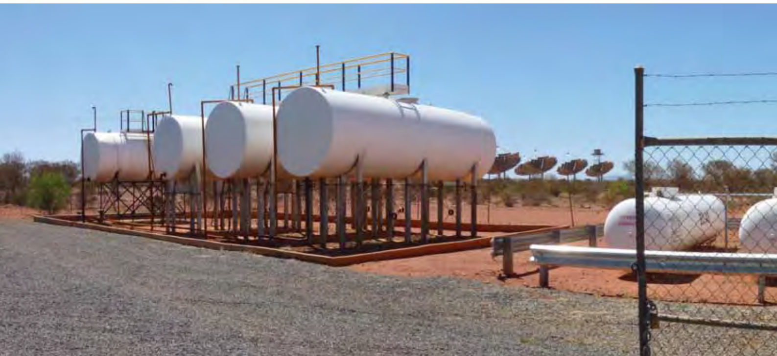
BELOW ► HERMANSBURG POWER STATION YARD
