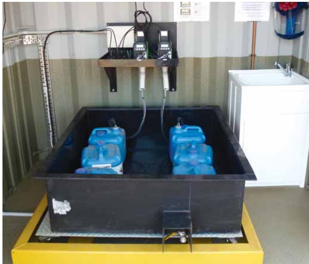
ABOVE: NEW DISINFECTION SYSTEM
