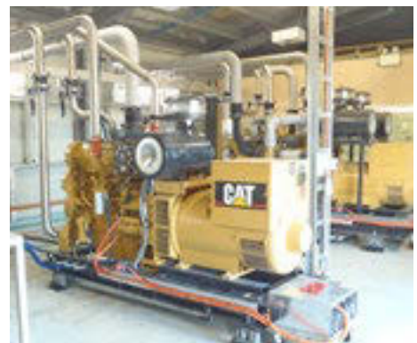
Each generator is maintained and checked daily by ESOs with major generator overhauls carried out by specialist contractors at regular intervals based on the number of operating hours.
