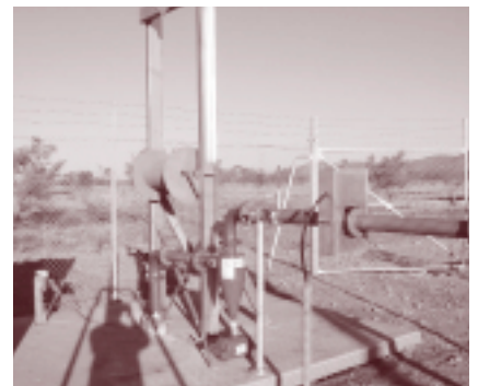
The Harts Range production bore.
