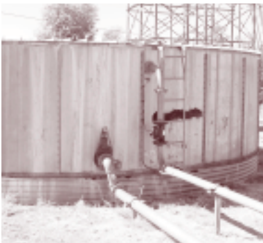
Old 120 KL Nyirripi ground tank.
