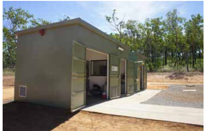
Gas Chlorination and Fluoride Plant at Wurrumiyanga
