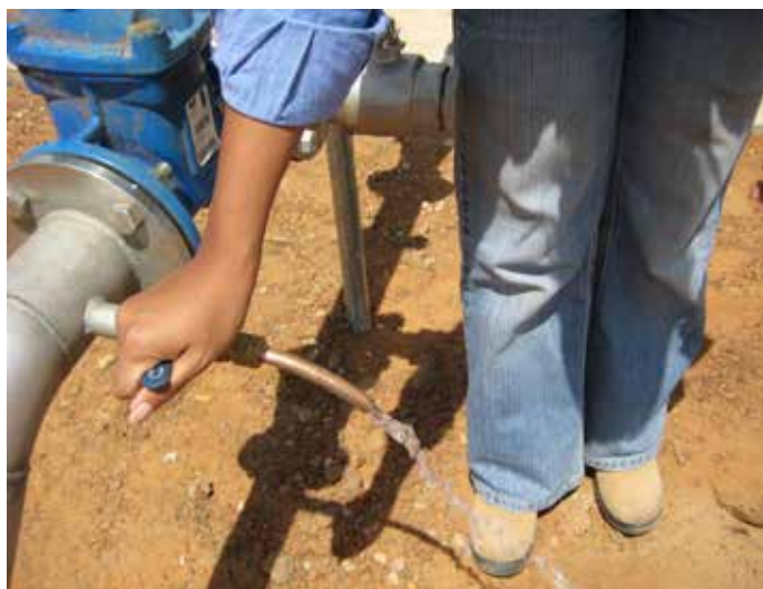
Water sample point on a production bore.
