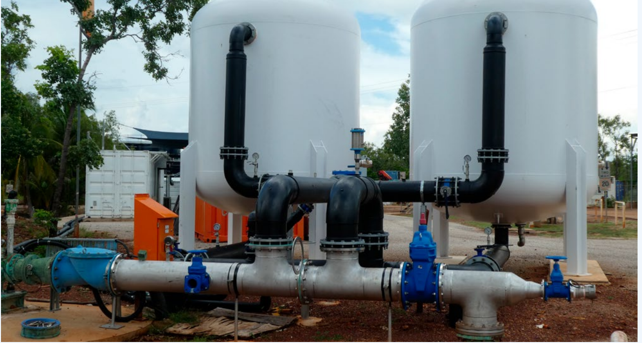
PFAS filtration vessels were temporarily installed in preparation for an emergency 'blackwater' event.
