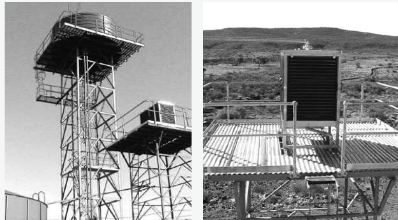
IMANPA AERATION UNIT.
