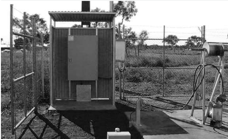
CANTEEN CREEK BOREFIELD SWITCHBOARD.
