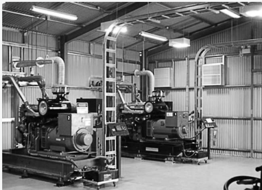
HARTS RANGE POWER STATION.
