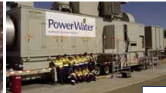
TITAN DUAL FUEL GAS TURBINE UNIT
