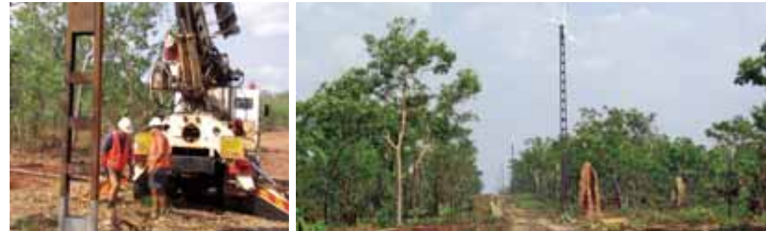
STAGE ONE OF THE DUNDEE BEACH POWER PROJECT
