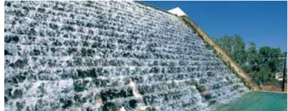
AERATION OF GROUND WATER AT THE KATHERINE WATER TREATMENT PLANT HELPS IMPROVE WATER QUALITY
