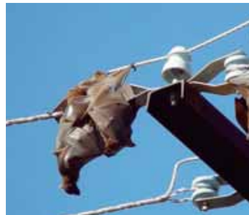
LONGER POST TOP INSULATORS ARE BEING INSTALLED TO REDUCE OUTAGES CAUSED BY BATS
