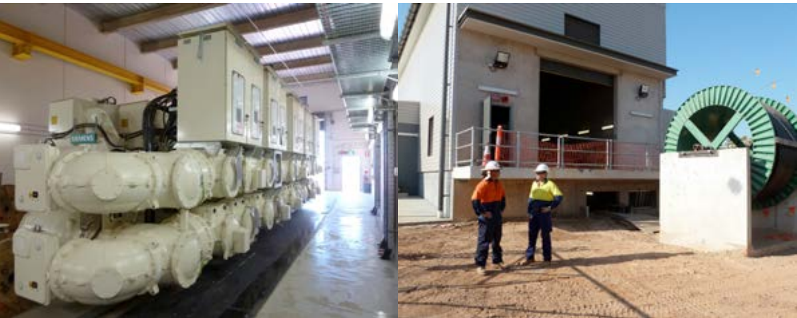
Darwin Zone Substation
