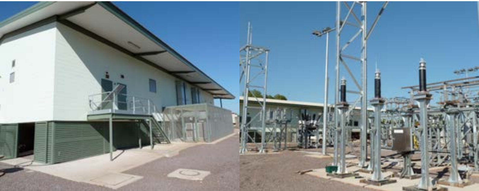
Leanyer Zone Substation
