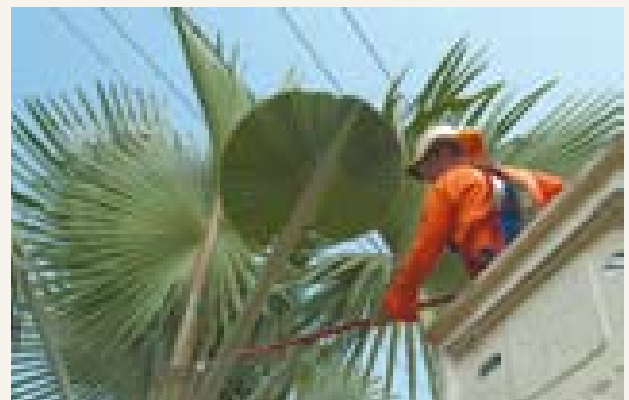
POWER AND WATER UNDERTAKES TREE-TRIMMING REGULARLY TO REDUCE VEGETATION AROUND POWERLINES.
