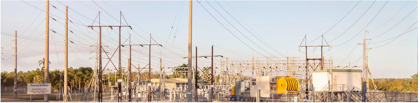
Hudson Creek substation
