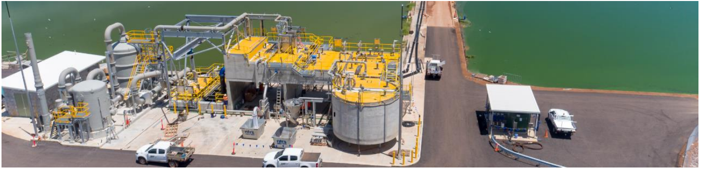
Leanyer Sanderson Waste Stabilisation Ponds Inlet Works
