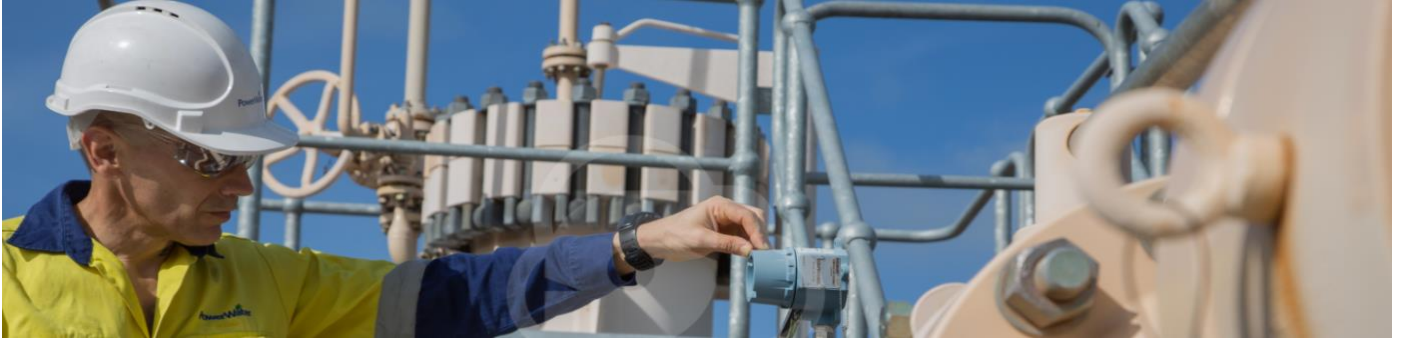
Gas infrastructure on Wickham Point pipeline
