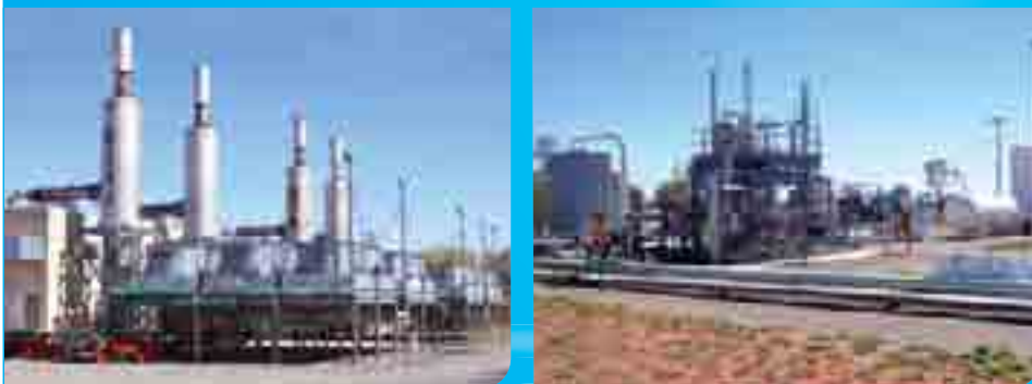
LEFT: YULARA POWER STATION AND GAS DELIVERY SYSTEM
