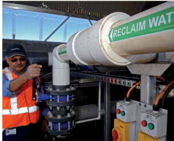
Alice Springs Water Reclamation Plant
