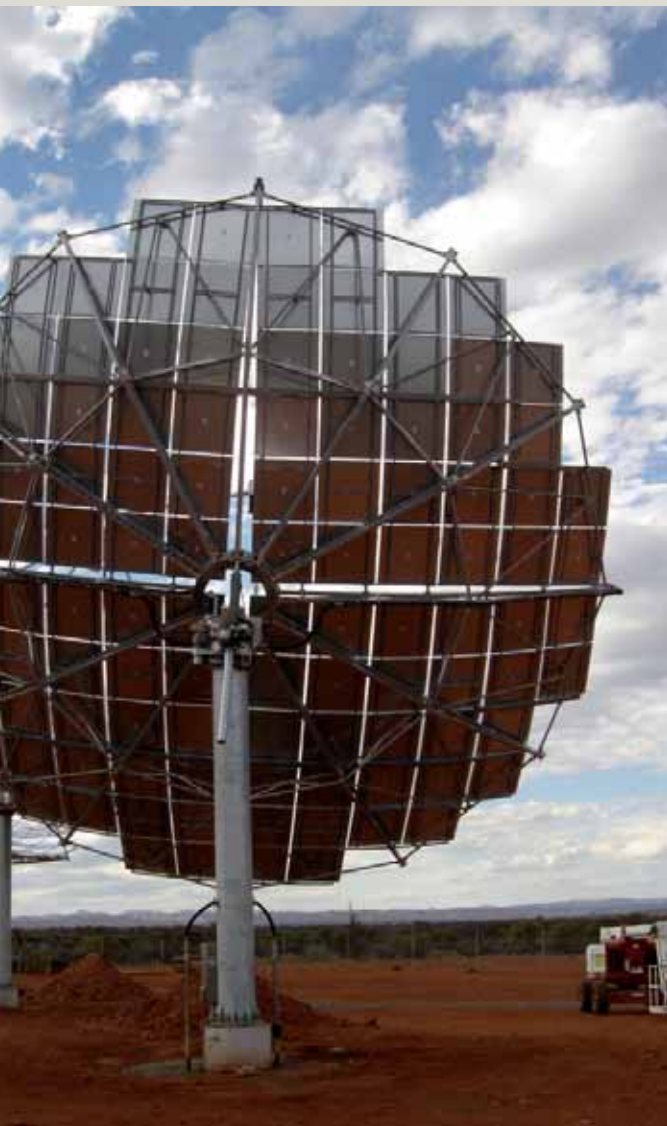
Solar panel at Ntaria
