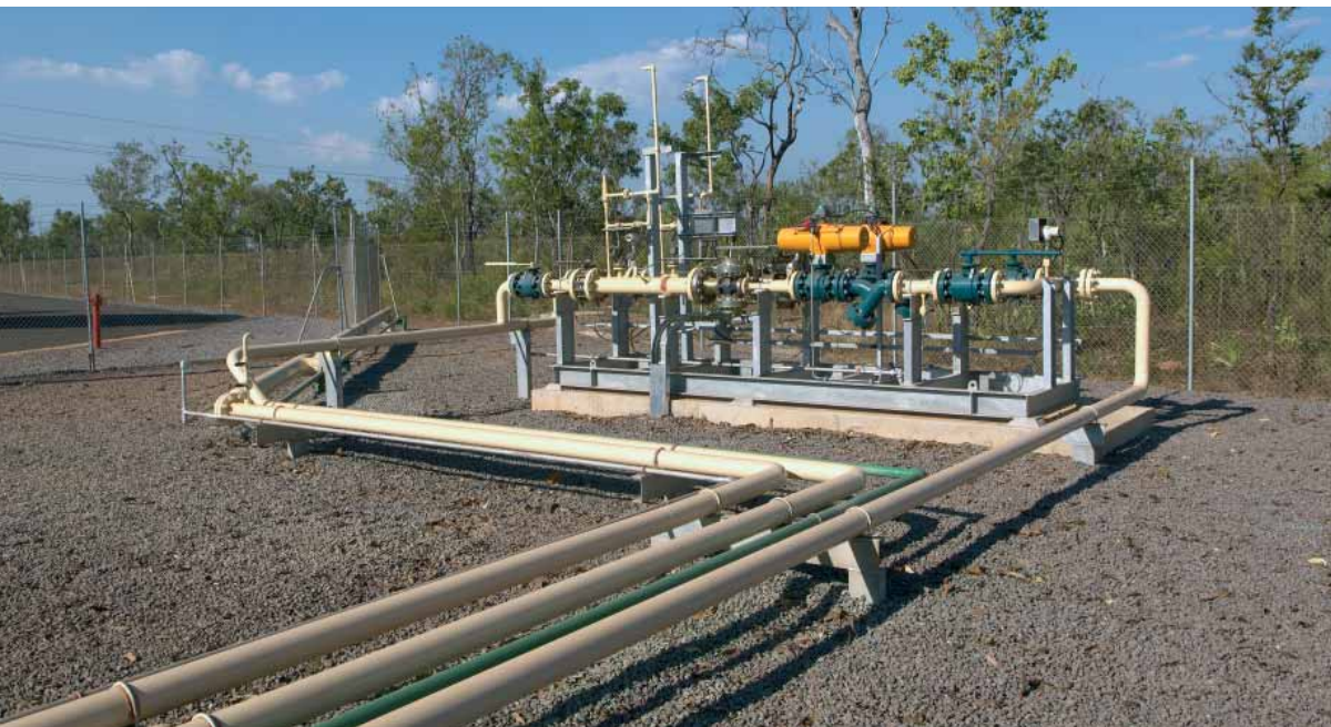
Pressure Reduction Skid for Weddell Power Station
