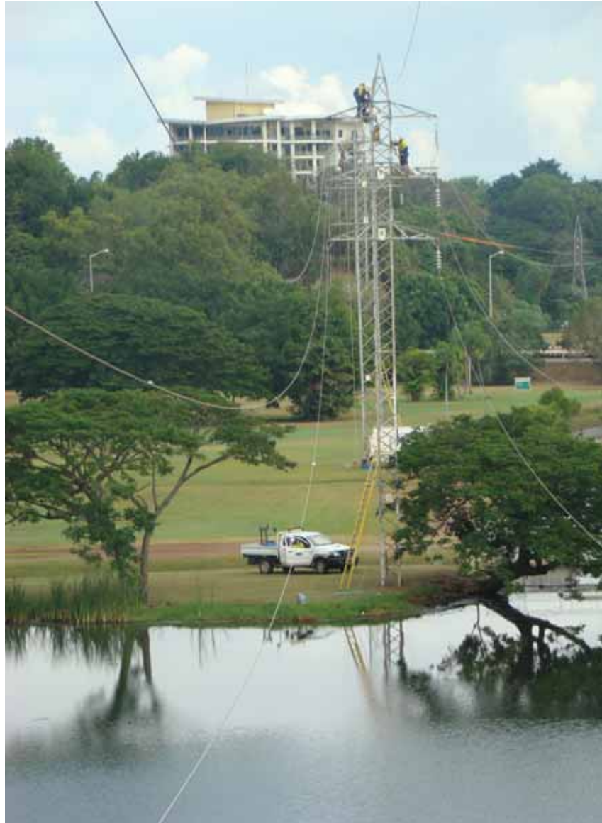
ABOVE ► POWER NETWORKS TEAMS WORKING ON LINES OVER GARDENS PARK GOLF COURSE IN DARWIN CITY
