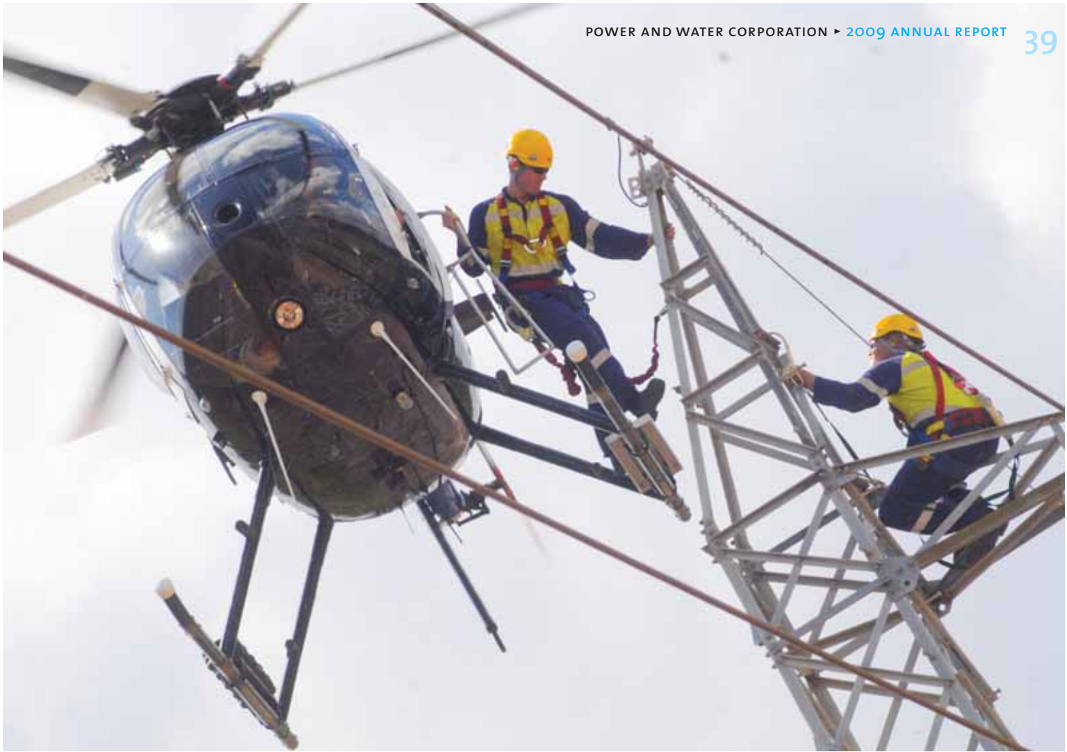
ABOVE ► POWER NETWORKS STAFF STEP FROM HELICOPTER TO POLE TO PERFORM LIVE WIRE MAINTENANCE.
