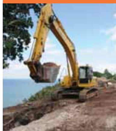
ABOVE ► EXCAVATION TO INSTALL A NEW SEWER ON LARRAKEYAH TERRACE AS PART OF THE LARRAKEYAH OUTFALL CLOSURE PLAN
