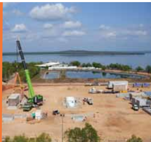
ABOVE ▶ ONE OF THE NEW ROLLS ROYCE TURBINES TO BE INSTALLED AT CHANNEL ISLAND POWER STATION
