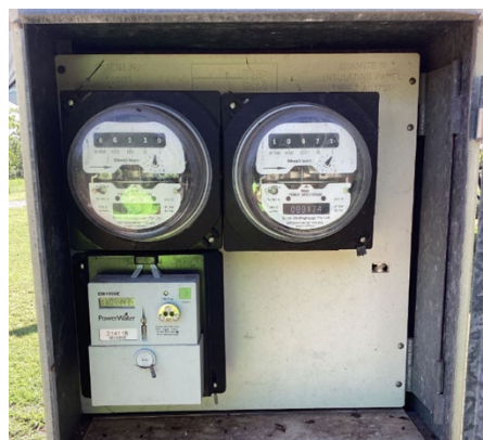
Figure 3.1: Example of three single phase meters
